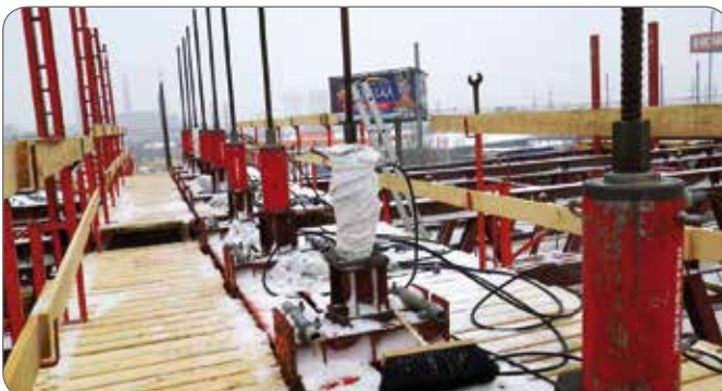
Lifting sections of concrete structure bridges using 60 ton-capacity hollow cylinders and traction bars.
